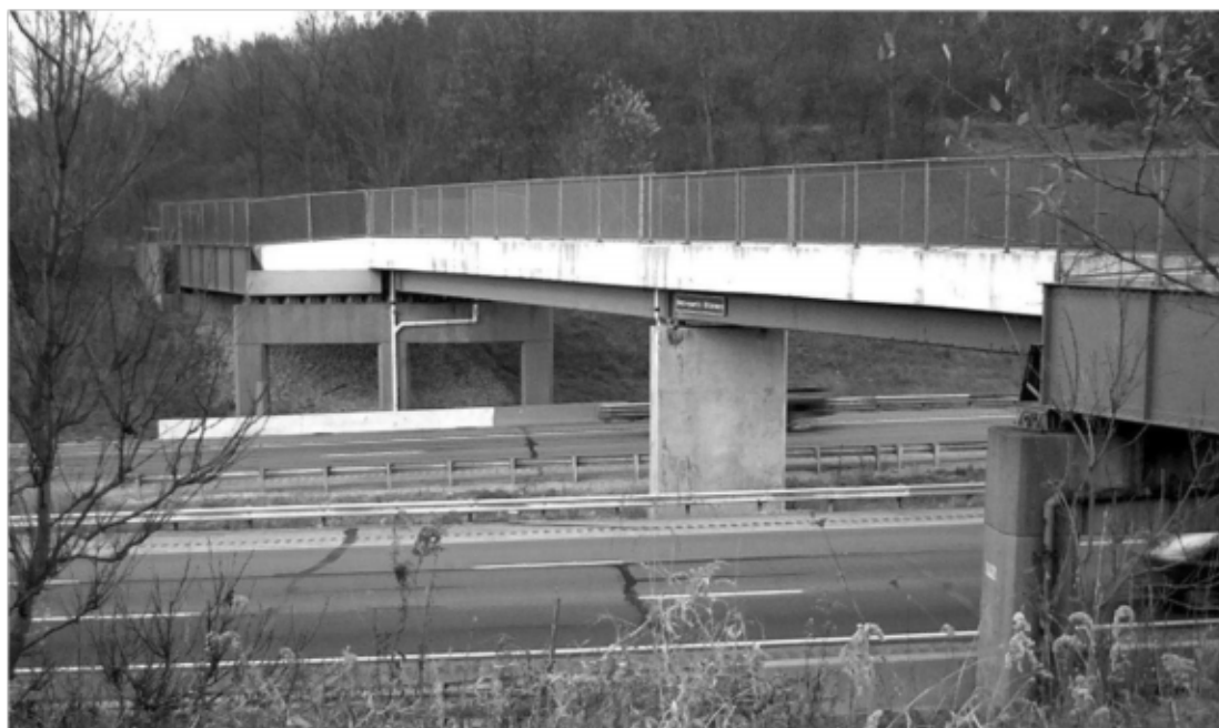
Rebuilt Bridge for Bike Trail over the Ohio Turnpike. Photo by Gene Stebbins
